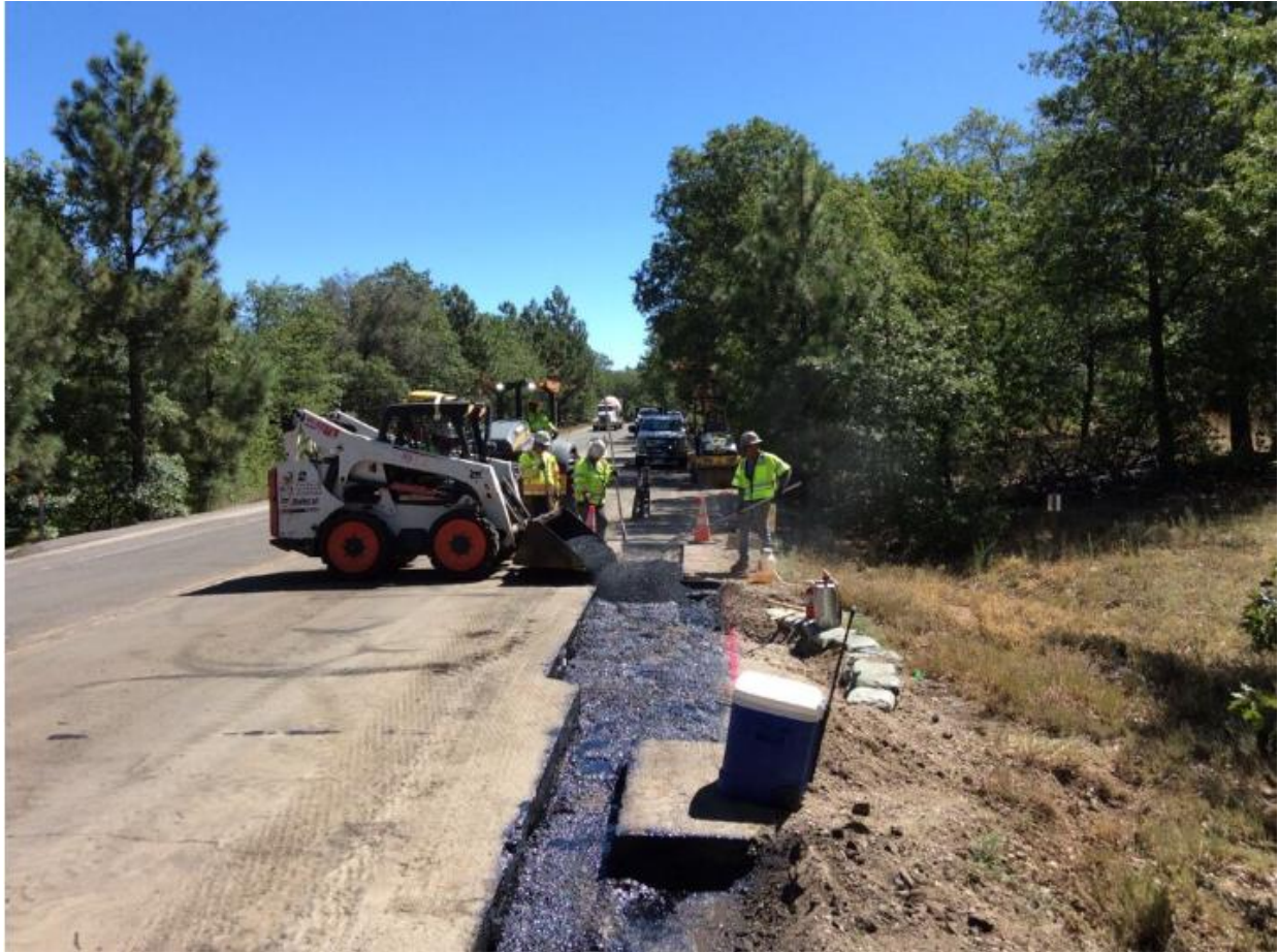
Photo 2: A crew was observed placing asphalt for paving the road near 444+50 (C 440).
