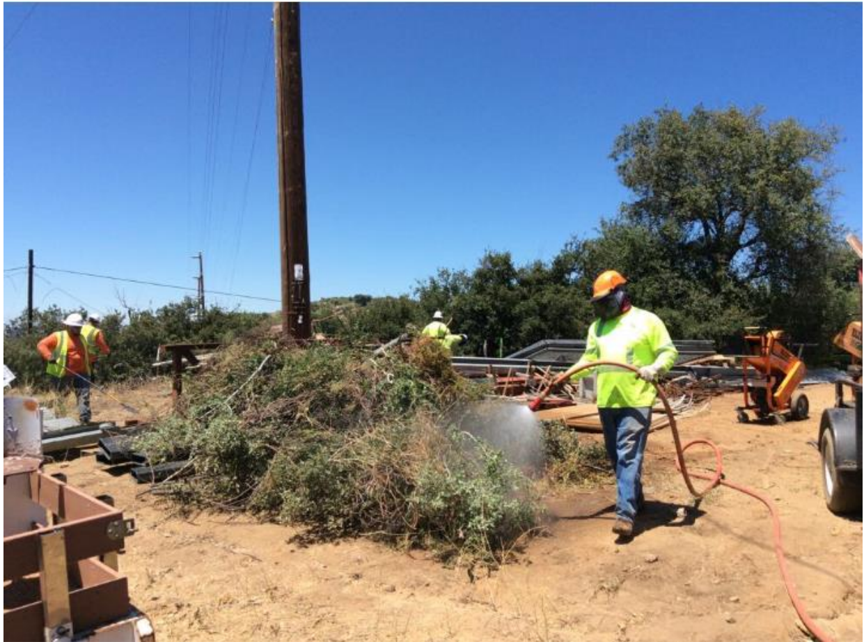
Photo 6: In accordance with the CFPPP matrix for the day's fire conditions (Elevated FPI off CNF land) vegetation was wet down prior to chipping at Pole Z173098 (TL 629A).
