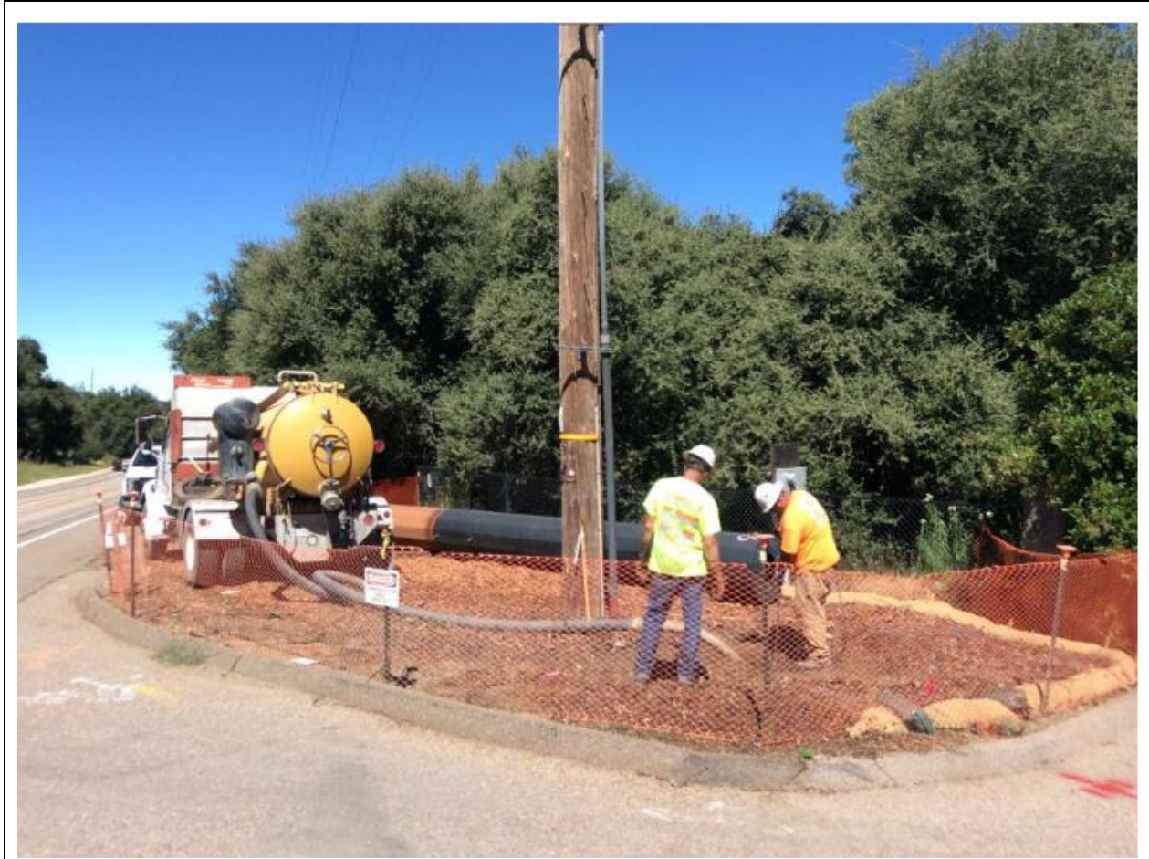
Photo 1: A crew was observed potholing for underground utilities at Pole Z173077 (TL 629A).
